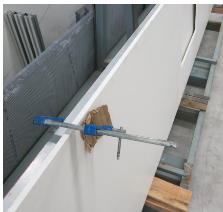
Image 3: Plank in the backside of the slab
